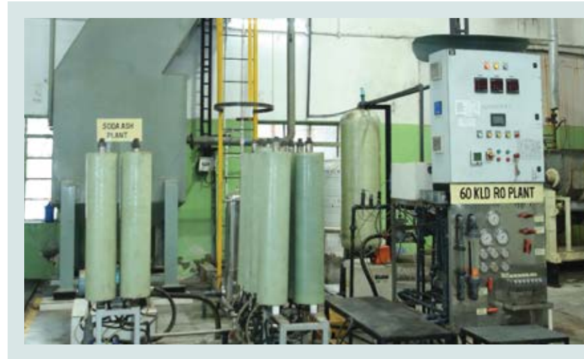
60 KLD RO unit
