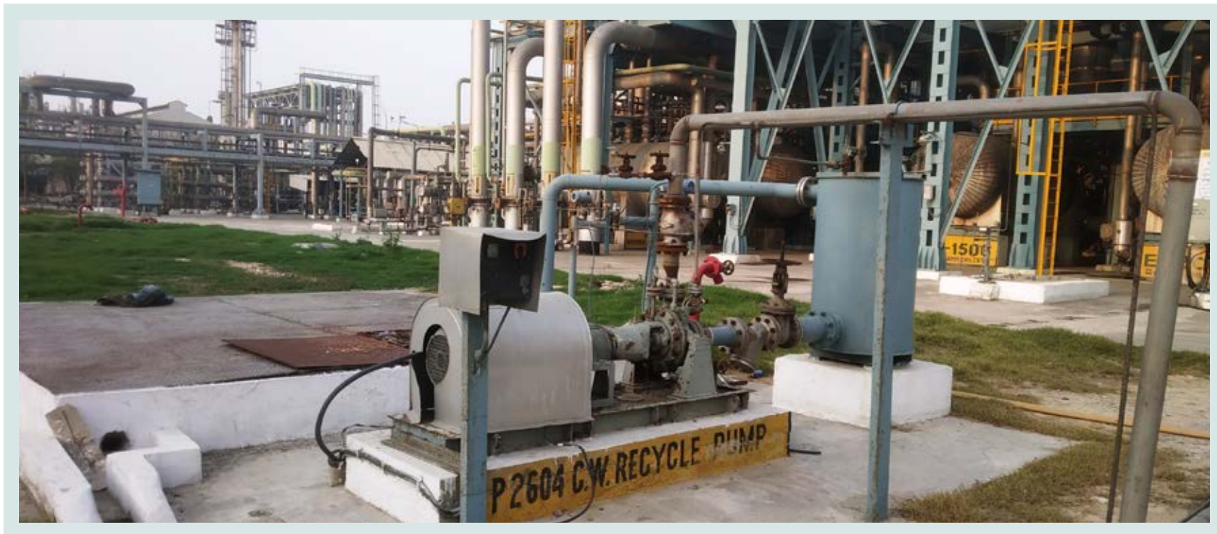
Cooling water return from lube oil / seal oil turbine bearings and condensate from gland condenser of compressor house is reused in Ammonia-I Plant as cooling tower make-up
