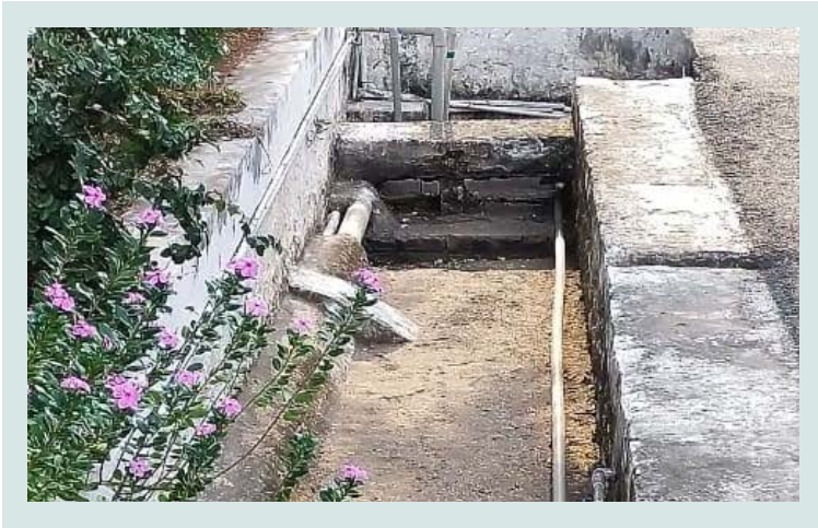
Trench Rainwater collection trench along plant periphery
