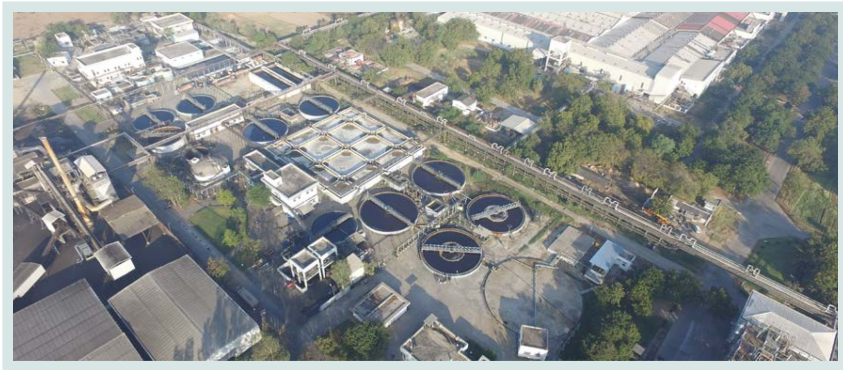
Effluent treatment plant
