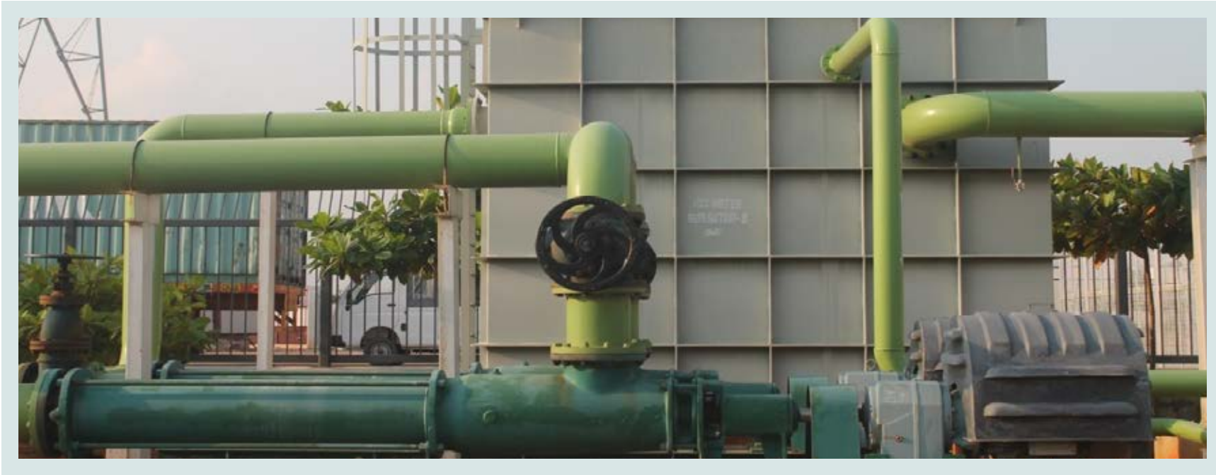
Oil water separator system
