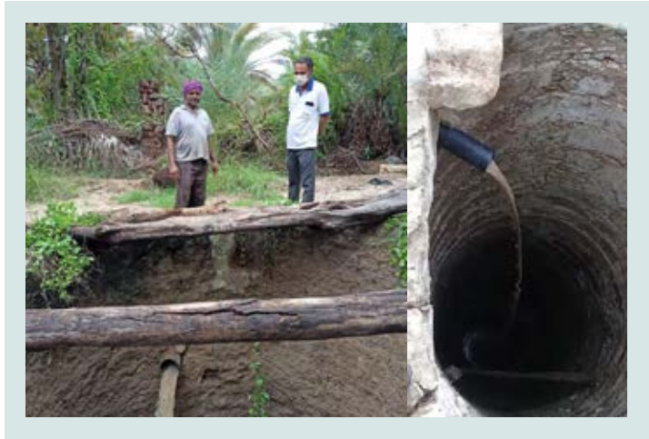
Artificial recharge through abandoned bore wells
