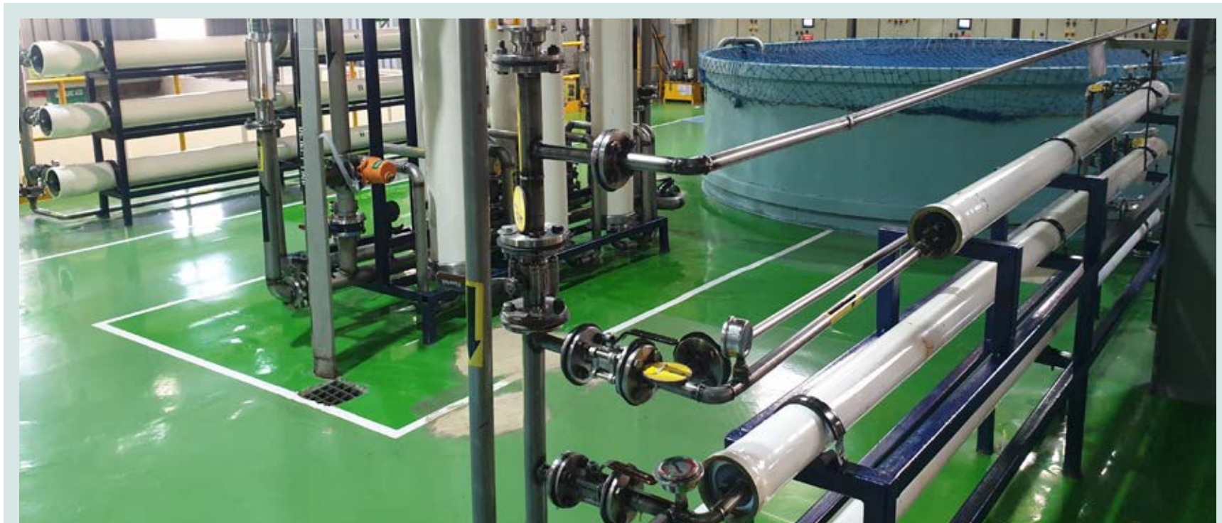
ETP Recycling Plant
