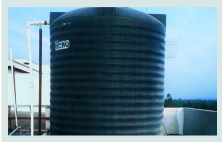
ETP treated water storage tank for toilet flushing
