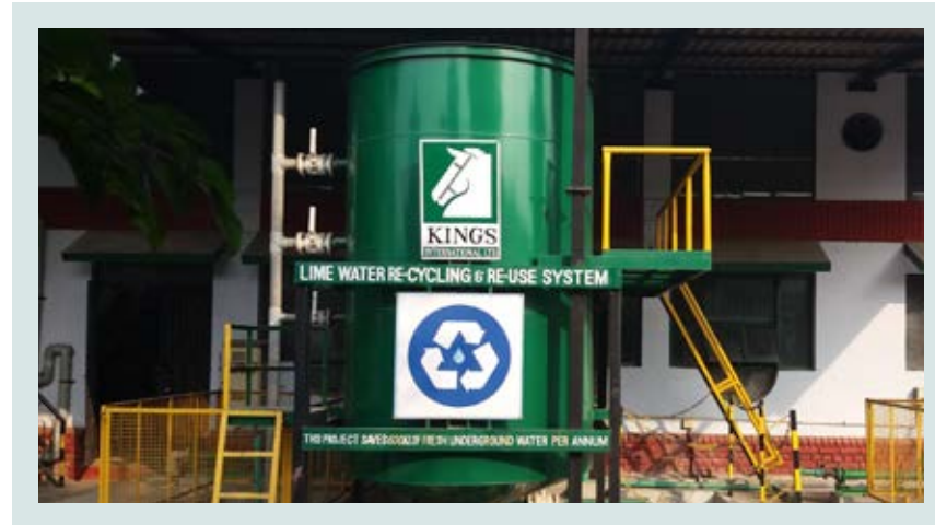
Lime Water Re-cycling & Reuse System
