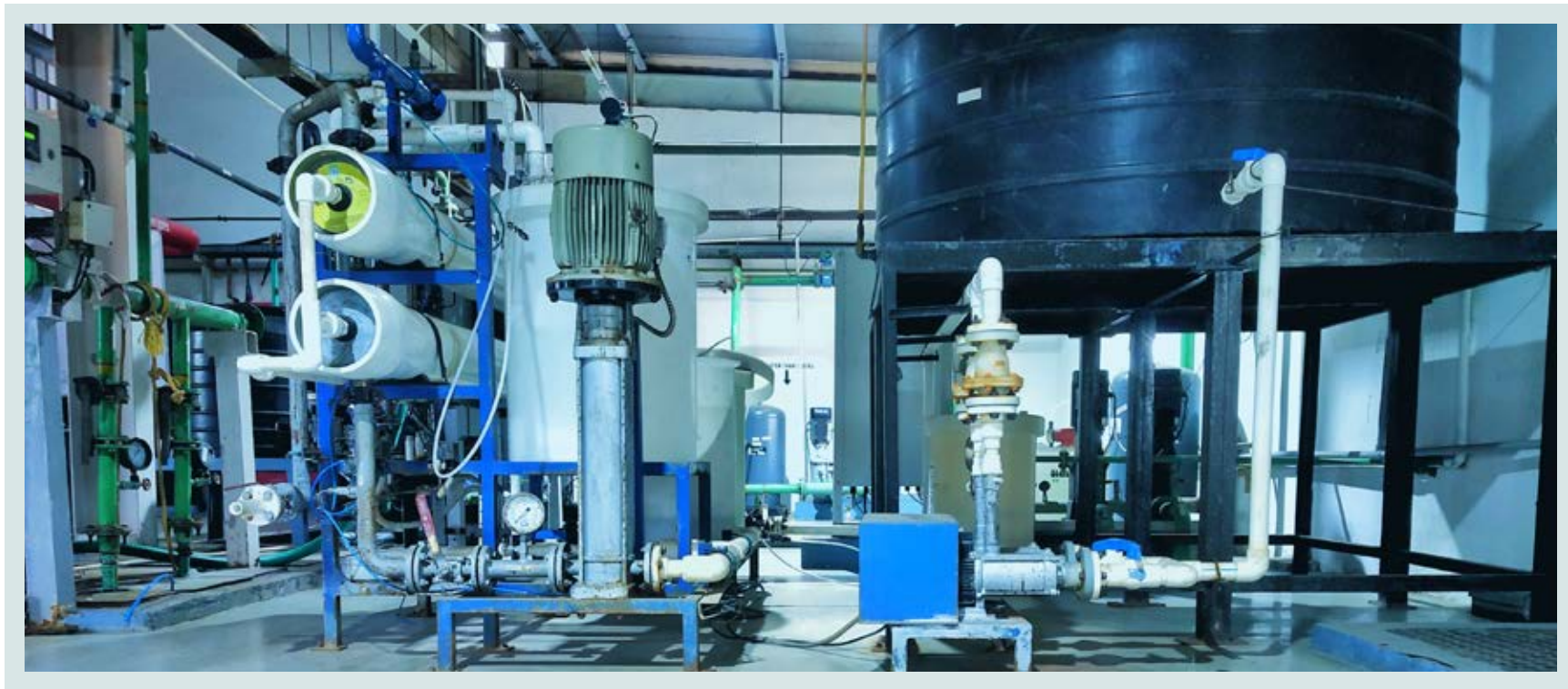
Second stage RO system installed in the water treatment plant to treat reject from first stage RO
