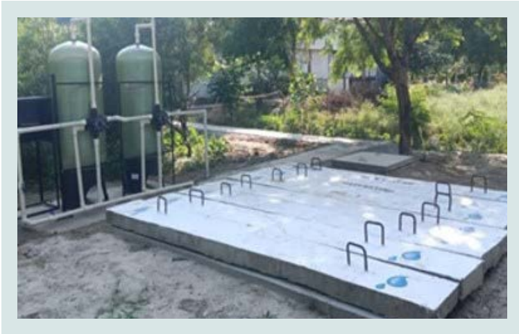
Roof top rainwater harvesting
