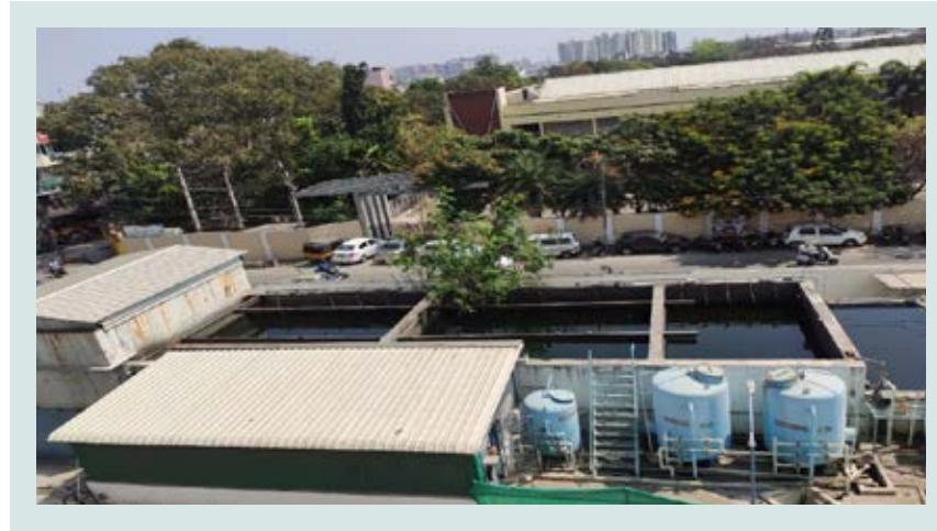
Sewage treatment plant at G.Kuppuswami Memorial Hospital, Coimbatore
