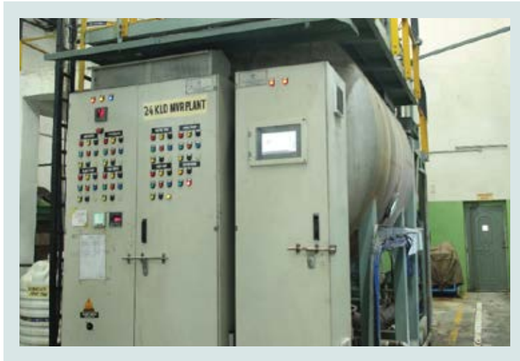
24 KLD MVR unit installed at the plant
