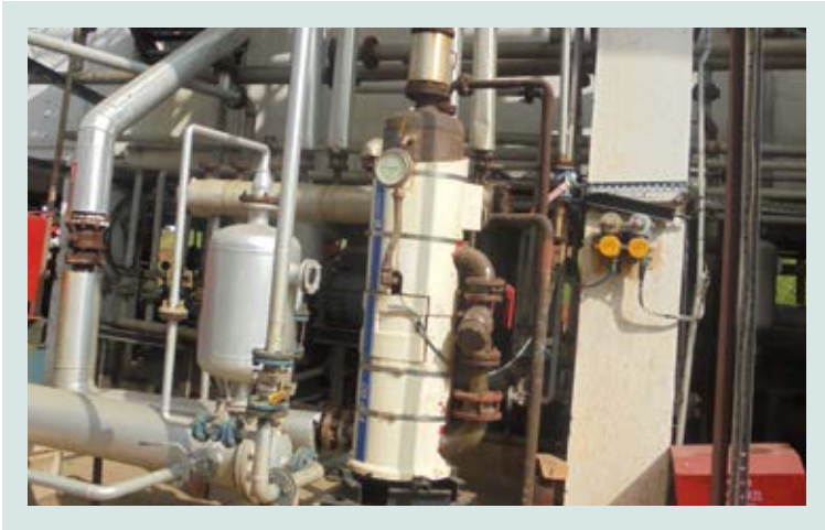
ATFD steam condensates recovered and flash steam reused in MEE stripper
