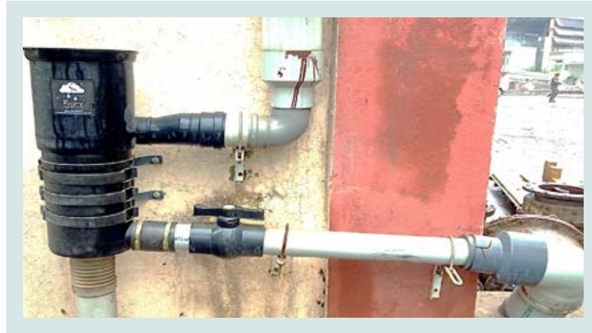
Roof Top Rain Water Harvesting
