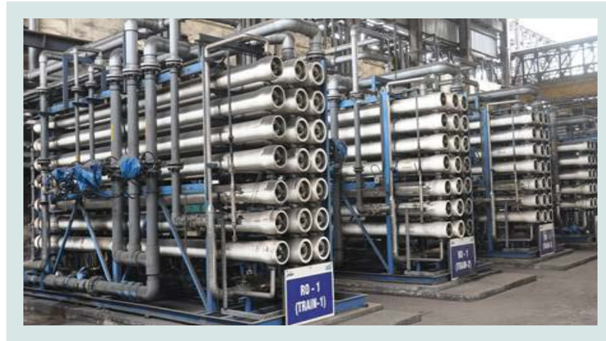
RO Plant at CRM-2
