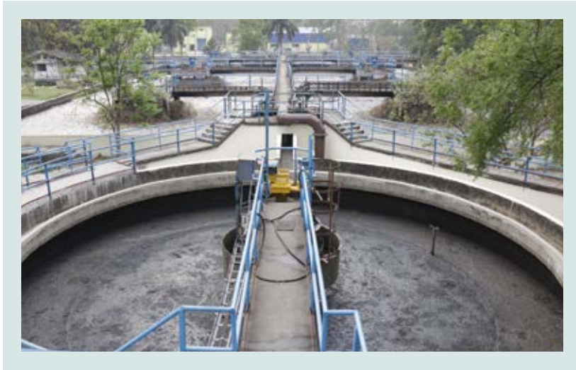
45MLD, Bara STP, Jamshedpur
