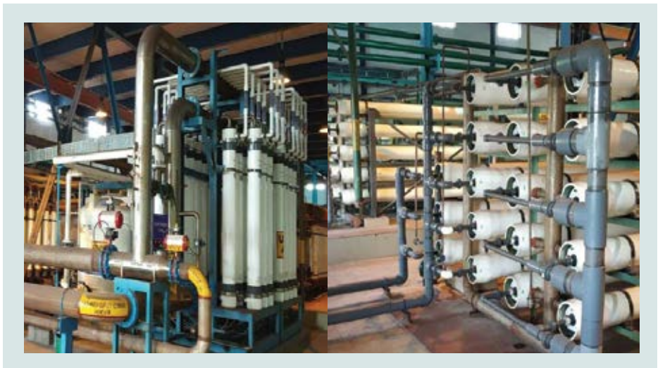
40 MLD Common Effluent Treatment Plant (Largest in India)
