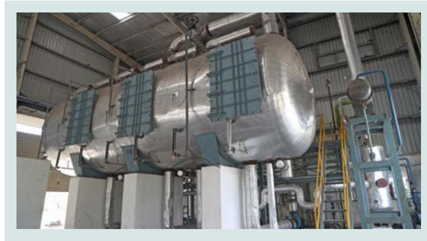
Mechanical vapor recompression evaporator
