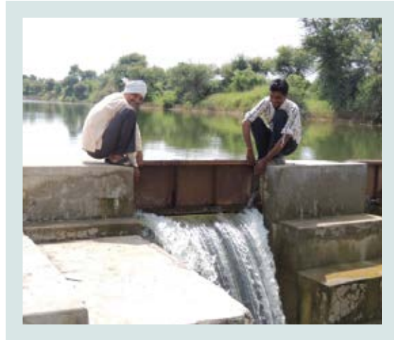
Water user group closing shutters of gated check dam for water conservation
