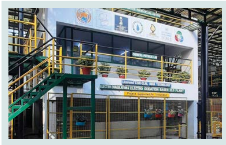
Electro Oxidation Plant
