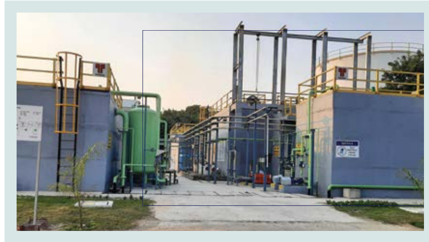
MBR based Sewage Treatment Plant with a capacity of 600m 3 / day
