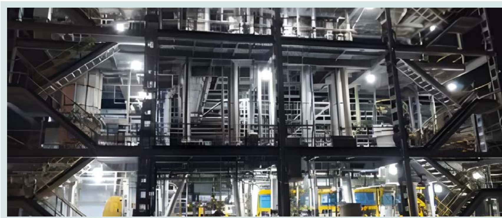
Sodium sulphate drying section 1
