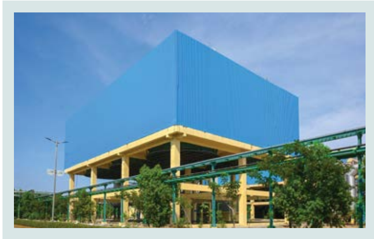
Air cooling at thermal power plant
