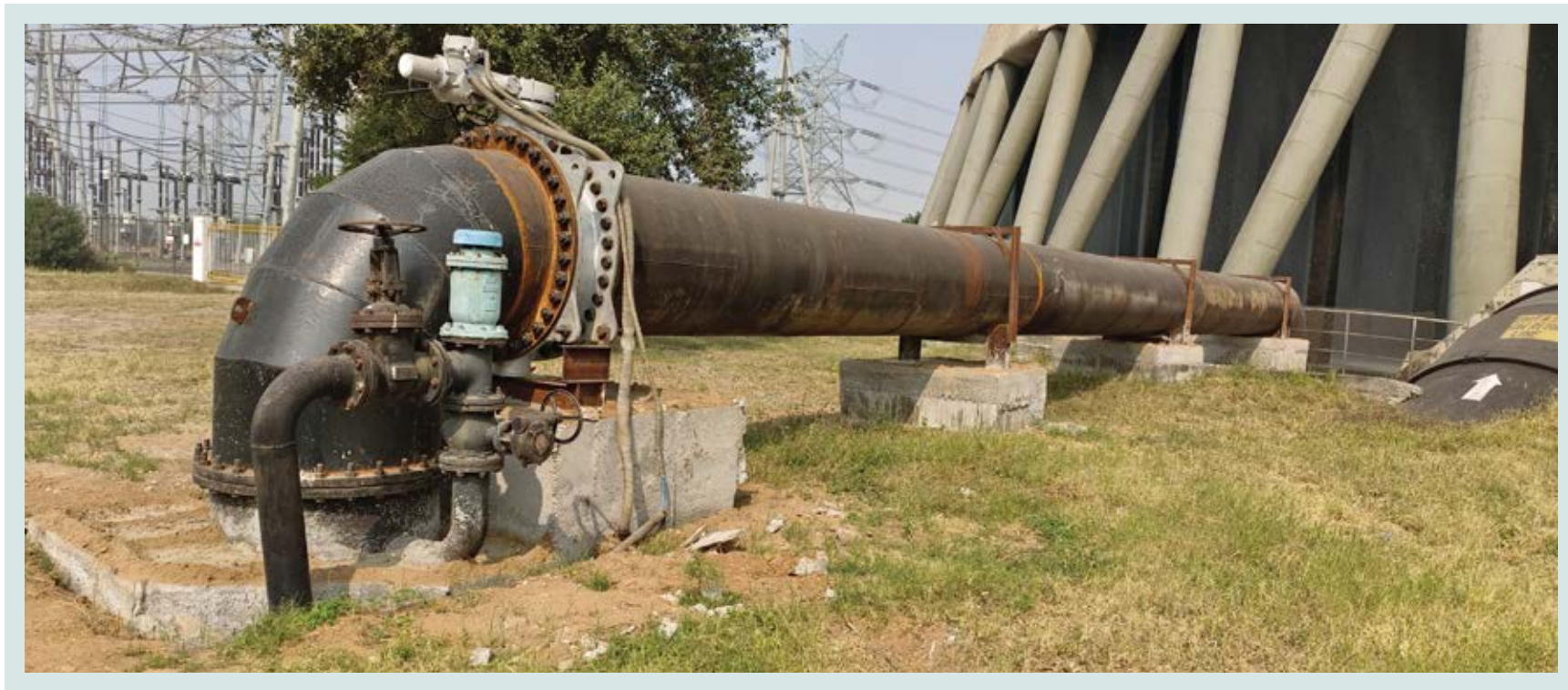
CW return line to sump to reduce evaporation loss
