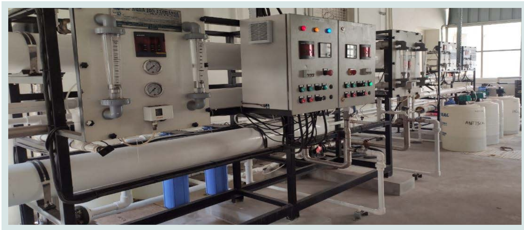
Four stage RO (ZLD - Zero Liquid Discharge), installed at G Kuppuswami Memorial Hospital, Coimbatore
