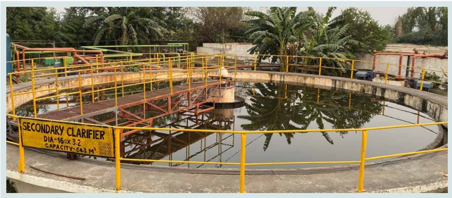
Secondary stage clarifier
