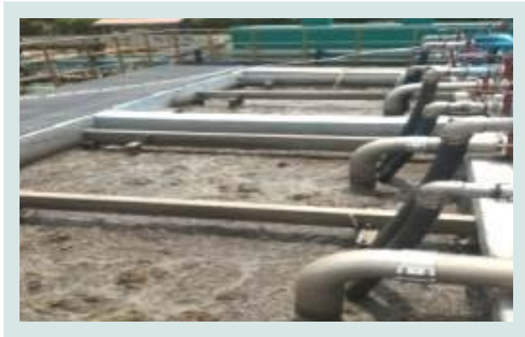
MBR Technology at Township STP
