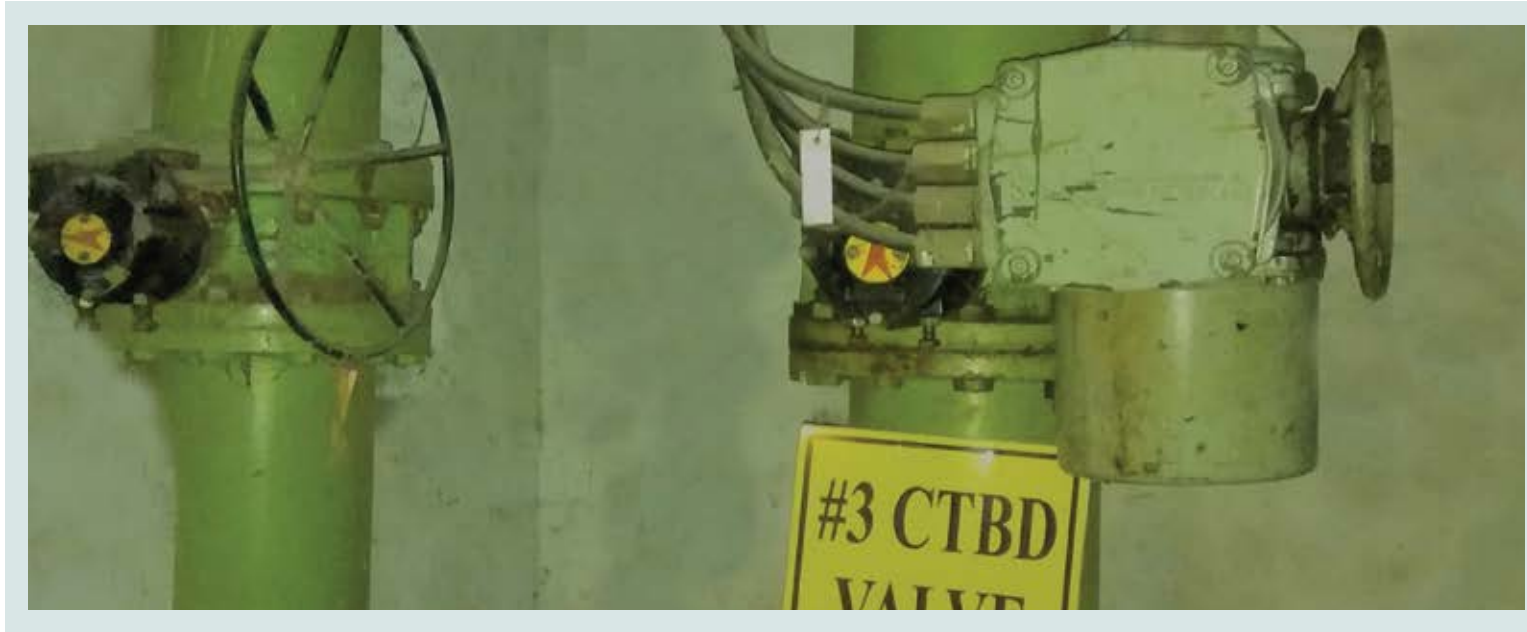
Cooling Tower Blow Down Valve
