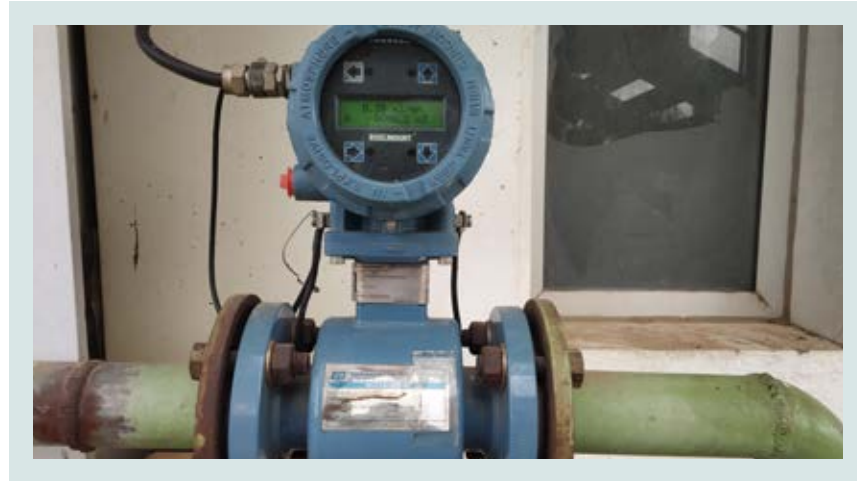
Water flowmeter for rest room
