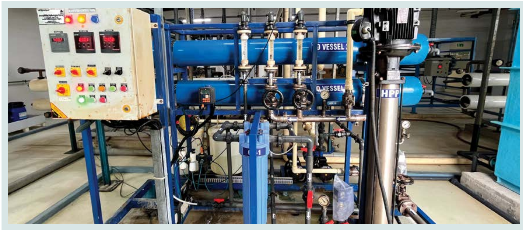
MEE condensate recovery plant
