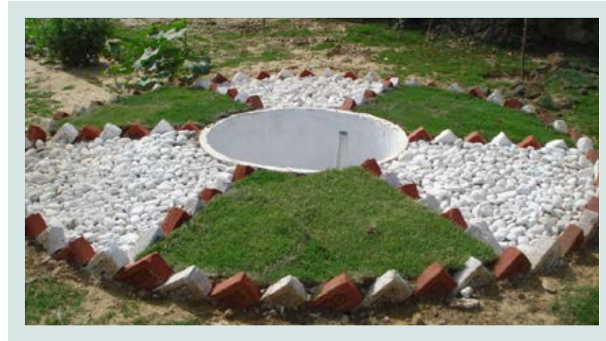
Rain water harvesting
