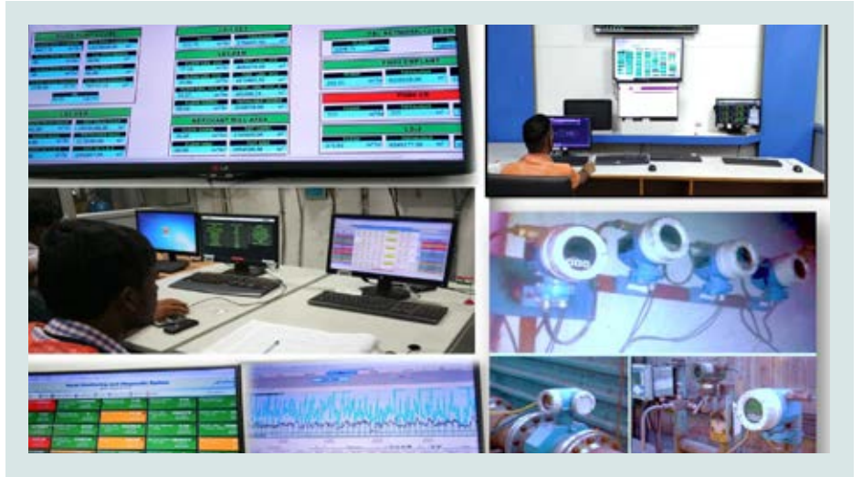
Water Management Central Station, Jamshedpur Steel Works
