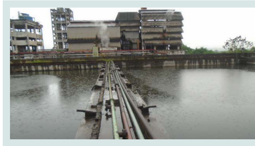
Rain water collection tanks
